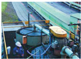
Froth flotation cells at Goedehoop Colliery are used for fine coal beneficiation.
